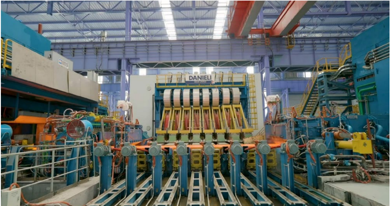
Fig.1 - Induction heating system between roughing and finishing mill stands.
