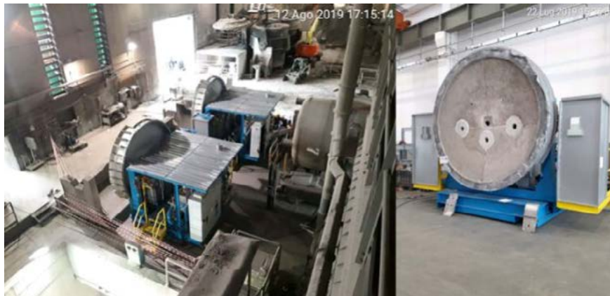
Fig.16 - New system for ladle preheating.
